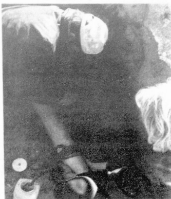
JIM WOOD AND Bill Rackley, Florida Gas Company, worked to stop the gas leakage Wednesday morning, Jan. 11. The leaking lines were located next to the tennis courts in Avon Park. Sunphoto by Mitch Banks.
