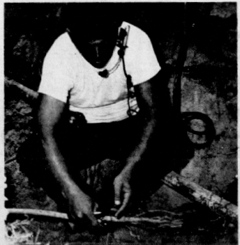
WORKMEN DIGGING A trench in the downtown area for placing underground gas pipe hit a buried telephone cable with four pairs of wires being cut and several having the insulation damaged. Butch Smith, working out of the Avon Park exchange is attaching alligator clips to wires to pick up the audible signal that indicates a pair of wires. Telephone service was restored in several hours. Photo—Miller.
