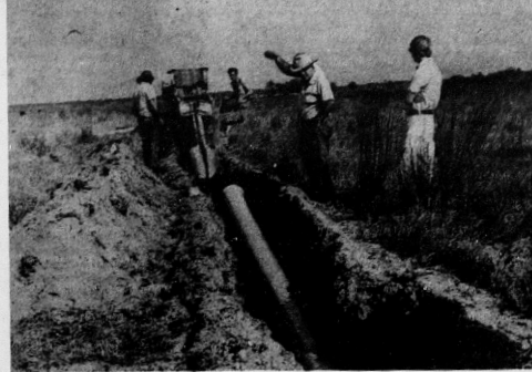
A TEN-INCH PLASTIC FEEDER line for a quarter mile long circular irrigation system. The A. A. Smith Ranch, Wauchula Rd., as Ed McClelland
