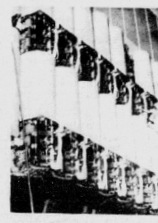
SWITCHMAN Tal Starr adjusts some of the additional local line switching equipment being placed into service for Avon Park subscribers by United Telephone next month. The equipment will add some 600 lines to the company's central office here.
